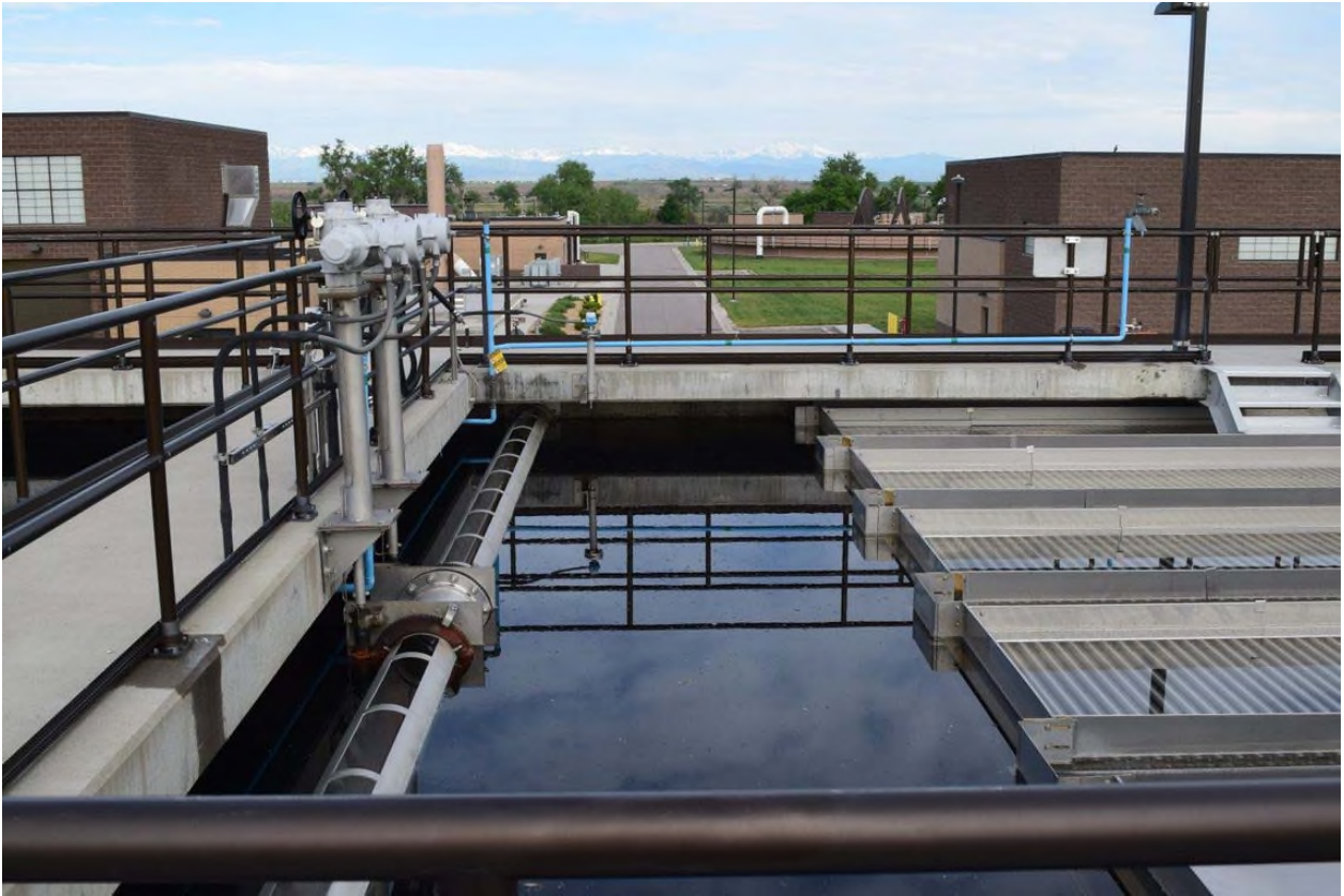
Northern Treatment Plant, taken in 2021
